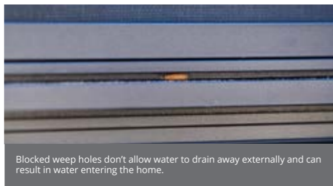
Check your weep holes are letting the water flow out freely and not overflowing.
