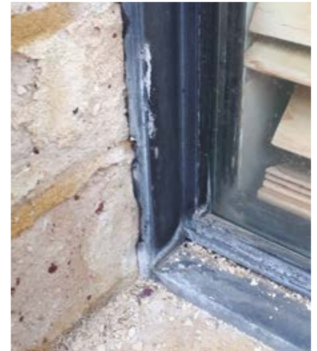
Regular cleaning and maintenance can greatly minimise the risk of salt damage and corrosion like this.
