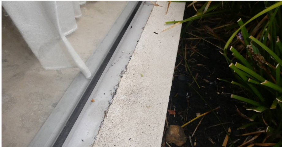
1. EARLY SIGNS OF CORROSION
