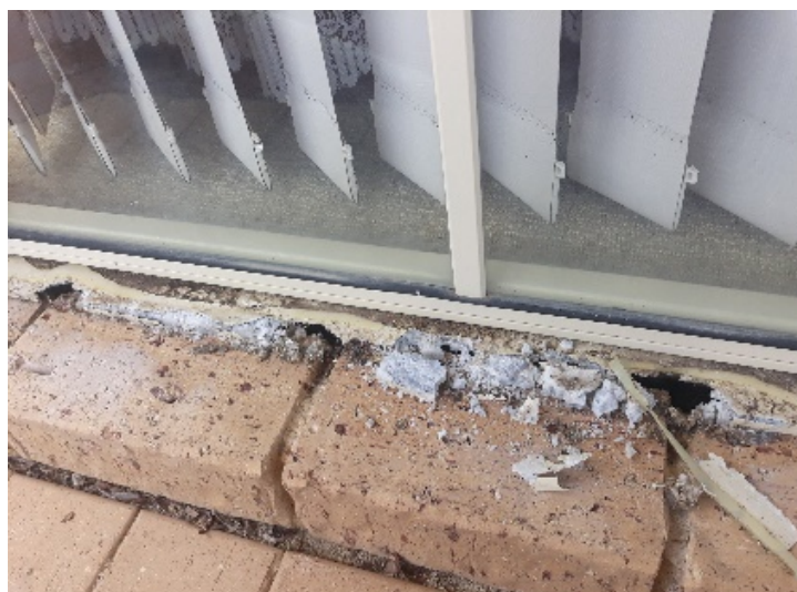
3 THIS IS WHAT CAN HAPPEN IF THE FIRST SIGN OF CORROSION IS LEFT UNTREATED
