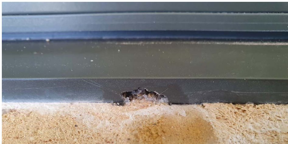
2. MOISTURE RISING FROM BRICKWORK OR LIMESTONE CAN CAUSE CORROSION OVER TIME
